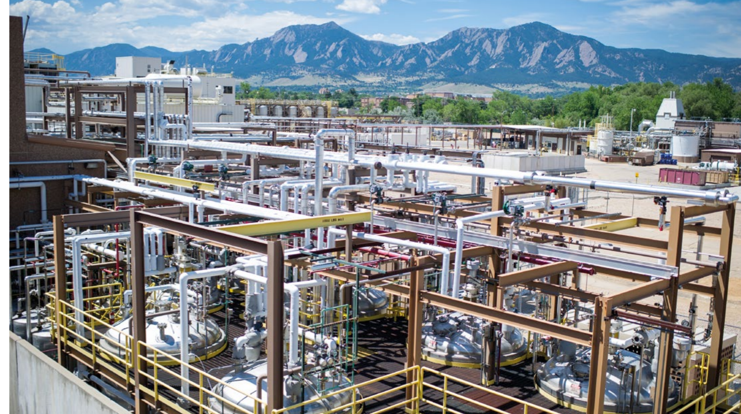
CordenPharma Colorado (USA) solvent handling infrastructure to support small molecule manufacturing.
